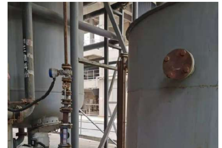
Sulfuric acid resin regeneration
